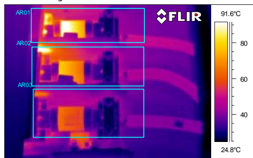
Delta "T" on inside of box of 33°C between phase "A" and "C".
